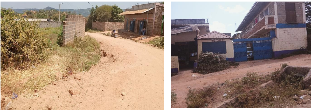
Figure 4-23: Narrow roads and clogging hinder effective storm water drainage
